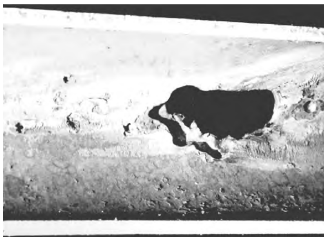
Fig. 2.19 Erosion–corrosion of a brass tube carrying out seawater. (Courtesy Defence R&D Canada-Atlantic.)
