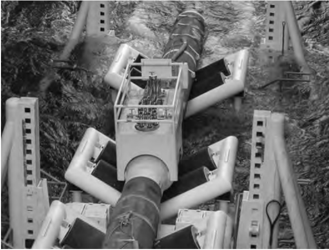
Fig. 4.9 A ring pair corrosion monitoring system being deployed at sea during the installation of a submerged pipeline. (Courtesy of Cormon Ltd.)
