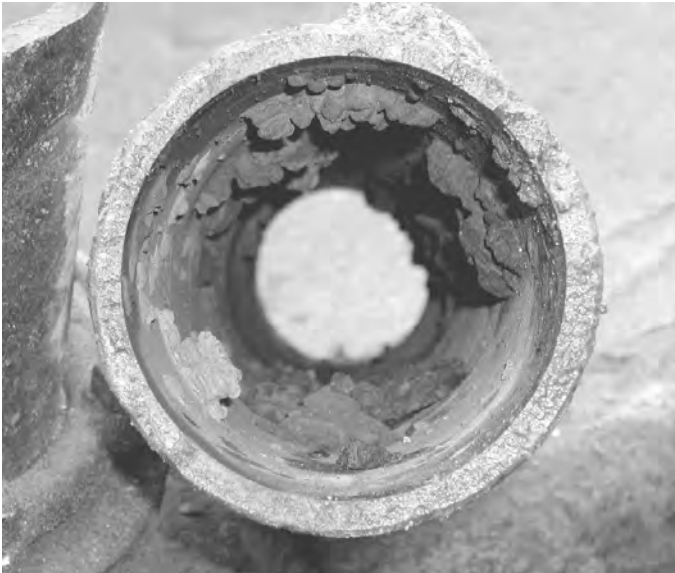
Fig. 3.32. Tubercles in a small diameter water pipe. (Courtesy Public Works and Services, City of Ottawa.)
