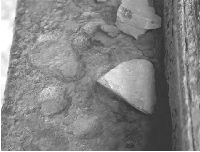
Fig. 2.12 Large holes created in a bridge structural steel by the presence of rocks. (Courtesy Kingston Technical Software.)
