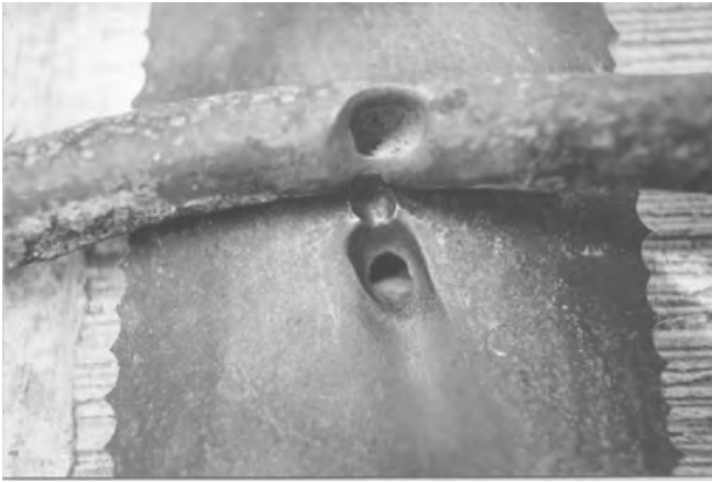
Fig. 2.4 Pits in the galvanized water pipe that contributed to the erosion corrosion of the gas line and the subsequent leak in a sewer main that caused the Guadalajara 1992 explosion (7). (Courtesy of Dr. Jose M. Malo, Electric Research Institute, Mexico.)
