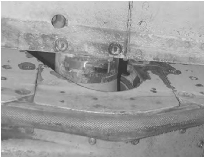
Fig. 2.20 Fretting corrosion at the interface of two highly loaded surfaces that are not designed to move against each other. (Courtesy Mike Dahlager Pacific Corrosion Control Corp.)
