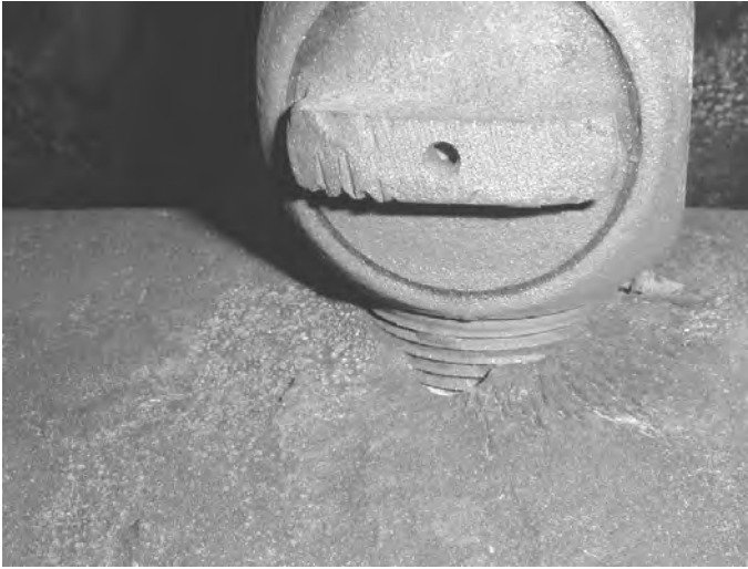
Fig. 2.16 Corrosion of a water main ductile iron adjacent to a copper fitting. (Courtesy Public Works and Services, City of Ottawa.)
