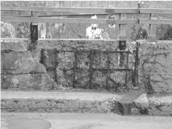
Fig. 1.9. Growth of the corrosion oxide products can lead to cracking and spalling of the concrete cover.
